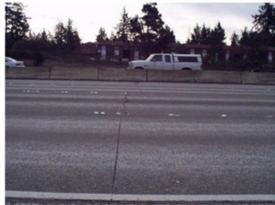
Figure 2.26: Missing Contraction Joint
